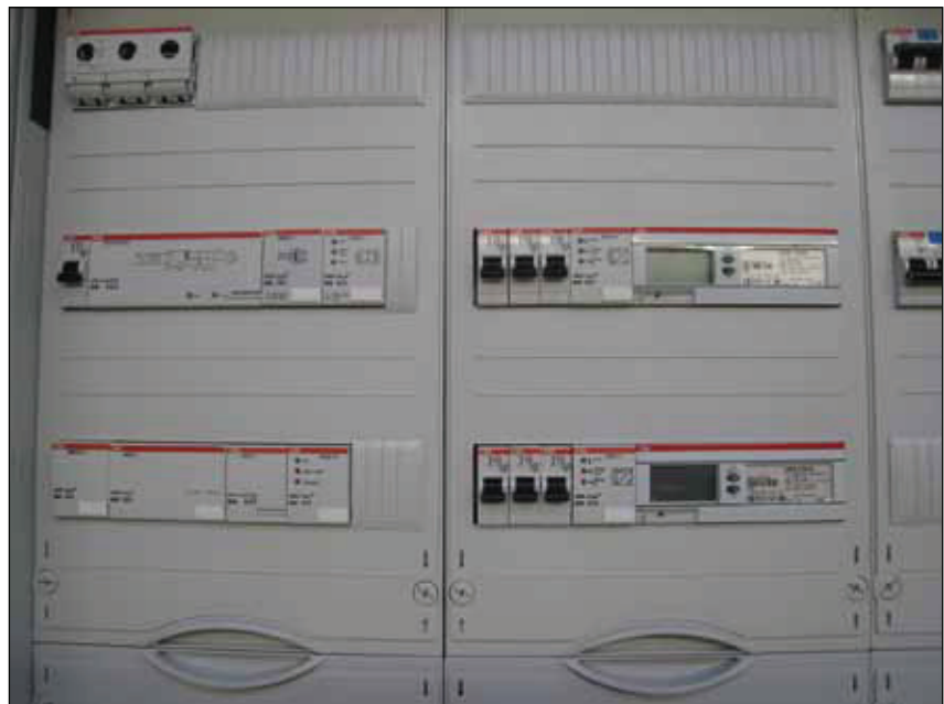
KNX Smart Metering
